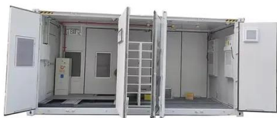
1075KW HH ESS
