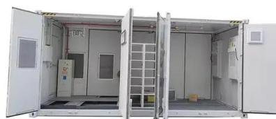
1075KW HH ESS
